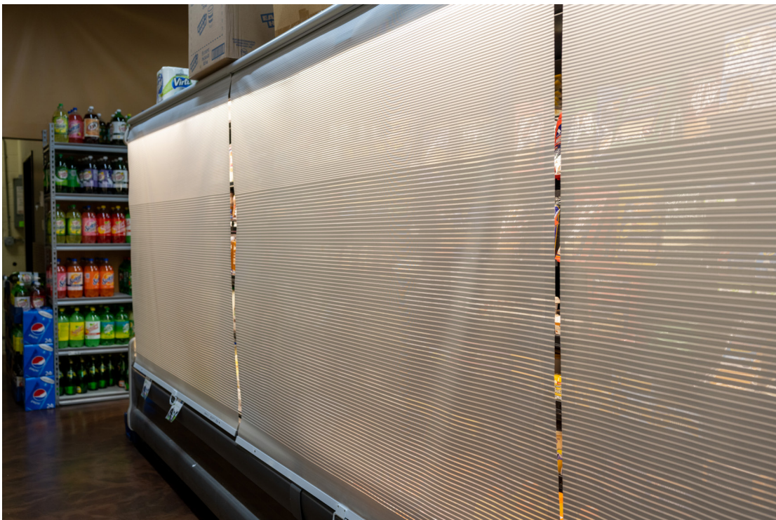
– Night covers on display cases to keep cold air from leaking
